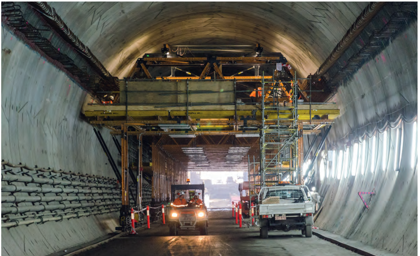
The self-propelled gantry built to support the drilling rig and workers on the Legacy Way Tunnel. PHOTO: HILTI
